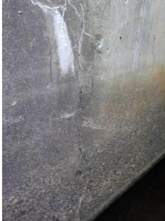
Crack in abutment
