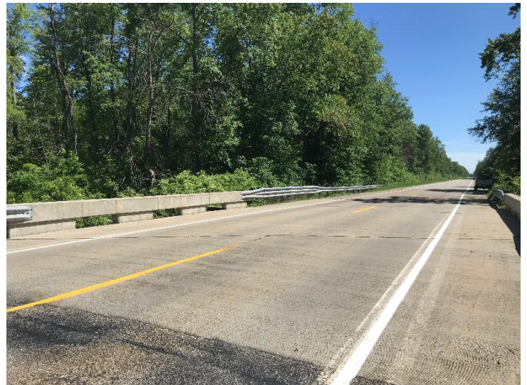
Document Name: IMG_2568.jpg Category: Deck Span Number: Comments: Looking south over structure
