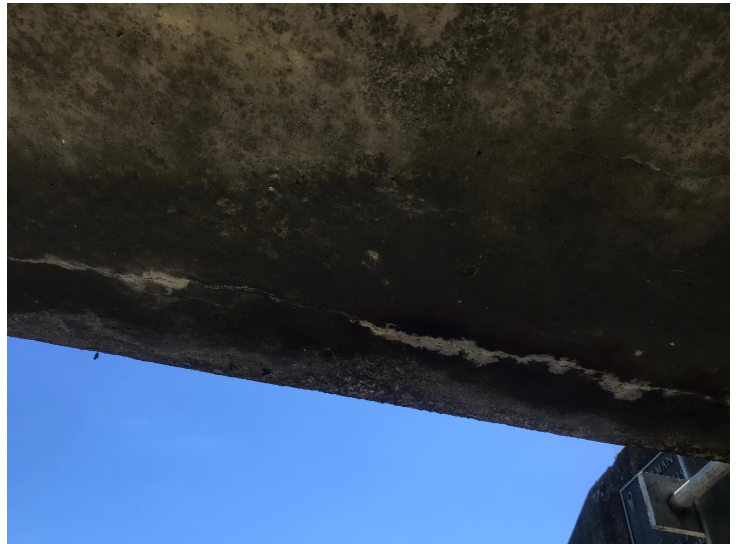
Document Name: IMG_2473.jpg Category: Superstructure Span Number: Comments: Longitudinal cracking with efflorescence along beam 1W
