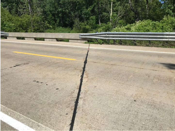
Document Name: IMG_2564.jpg Category: Joints Span Number: Comments: South reference line joint
