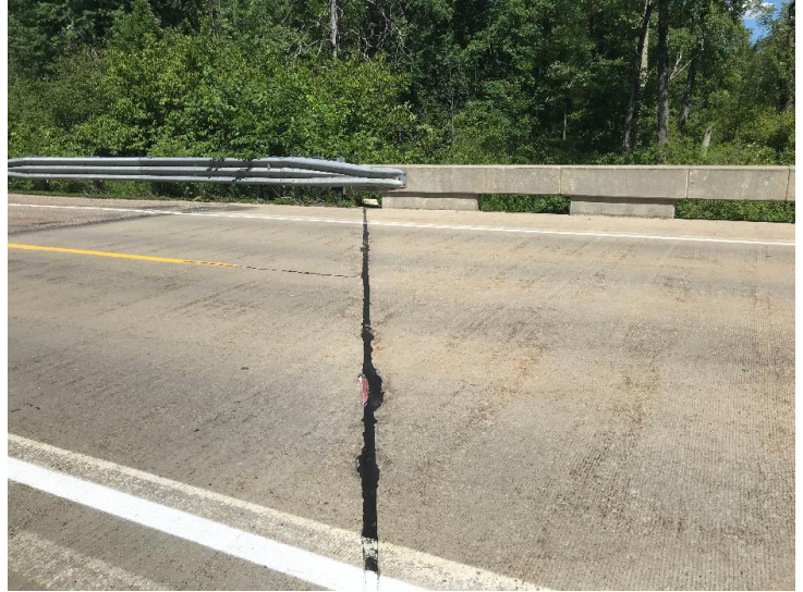
Document Name: IMG_2566.jpg Category: Joints Span Number: Comments: North reference line joint
