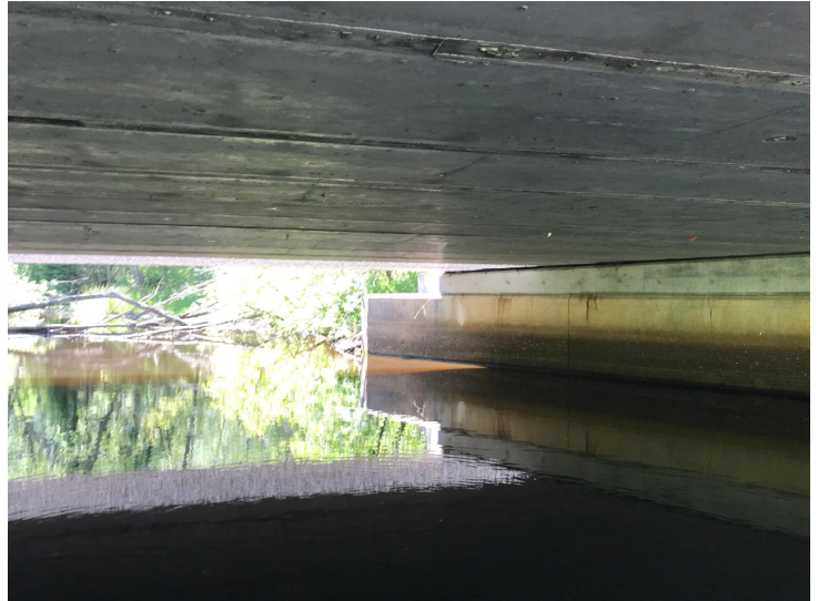
Document Name: IMG_2575.jpg Category: Superstructure Span Number: Comments: Prestressed concrete box beams
