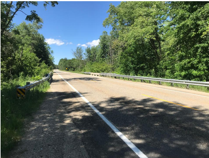
Document Name: IMG_2562.jpg Category: Deck Span Number: Comments: Looking north over structure
