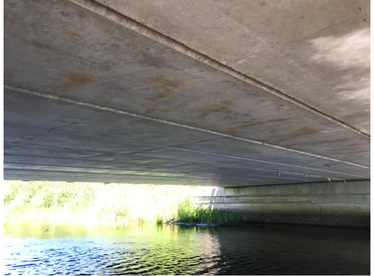
Document Name: IMG_2478.jpg Category: Superstructure Span Number: Comments: Prestressed concrete box beams
