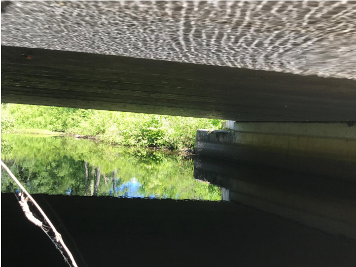
Document Name: IMG_2571.jpg Category: Superstructure Span Number: Comments: Prestressed concrete box beams
