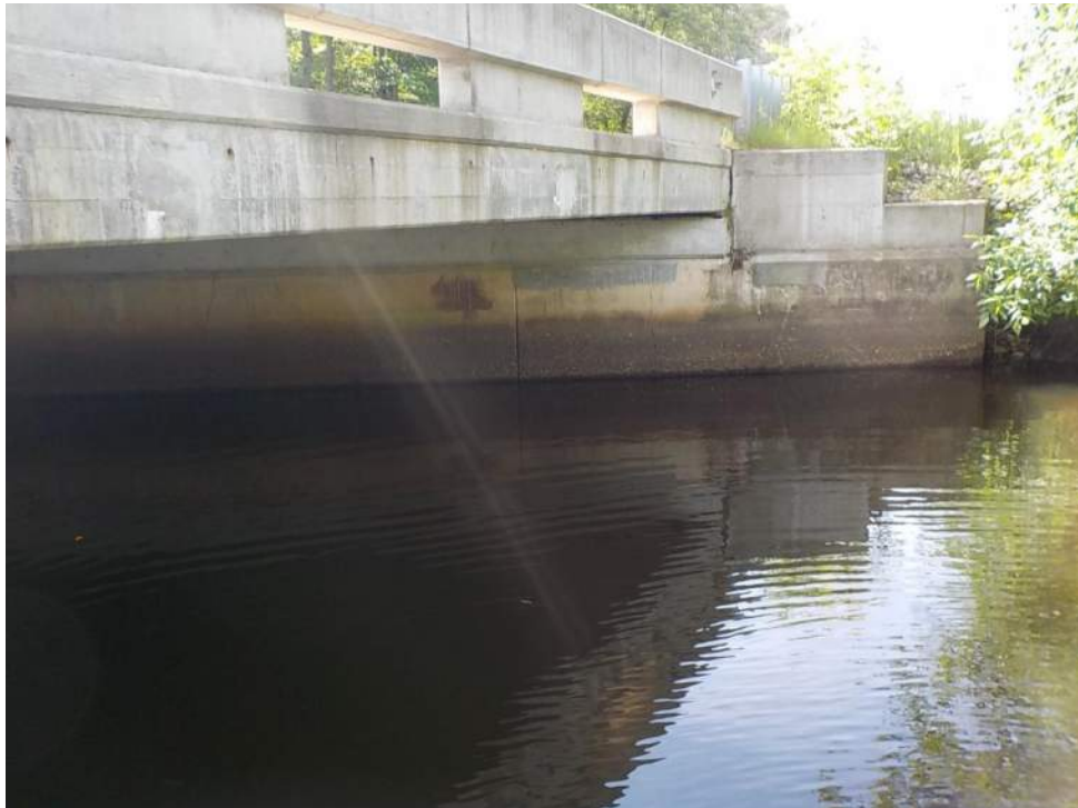
Cracking in abutment and slopewall
