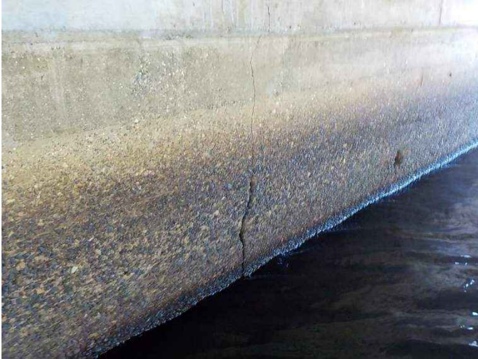
Crack in abutment
