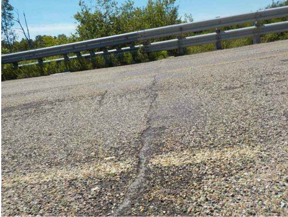
Cracking in HMA surface
