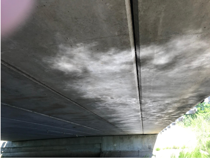
Document Name: IMG_2477.jpg Category: Superstructure Span Number: Comments: Prestressed concrete box beams
