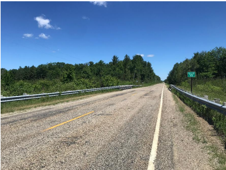
Document Name: IMG_2466.jpg Category: Deck Span Number: Comments: Looking north over structure
