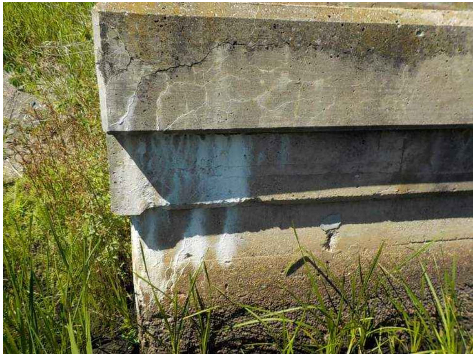
Cracking with efflorescence in sloped wall
